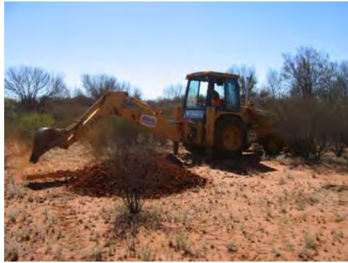
PHOTOGRAPH G4.1 John Deere 315D backhoe used to excavated test pits at Mount Everard and Harts Range site (photographed at Harts Range)
