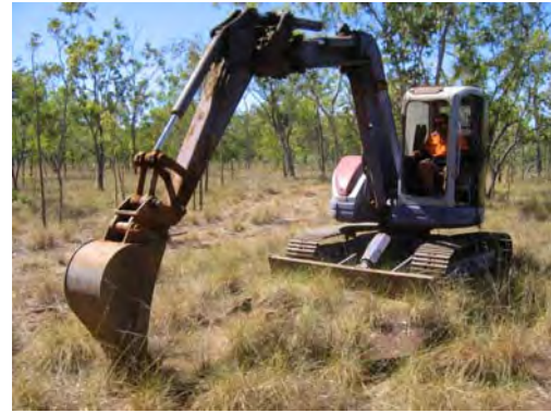
PHOTOGRAPH G4.2 Komatsu PC75UU tracked excavator used to excavate test pits at Fishers Ridge site
