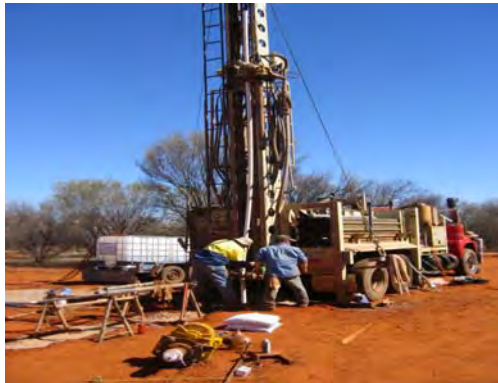
PHOTOGRAPH G4.5 Installation of groundwater monitoring well with Class 18 PVC standpipe (MEBH01)
