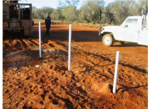
PHOTOGRAPH G4.8 50 mm non-slotted PVC standpipe used for the FHT tests at HRBH01
