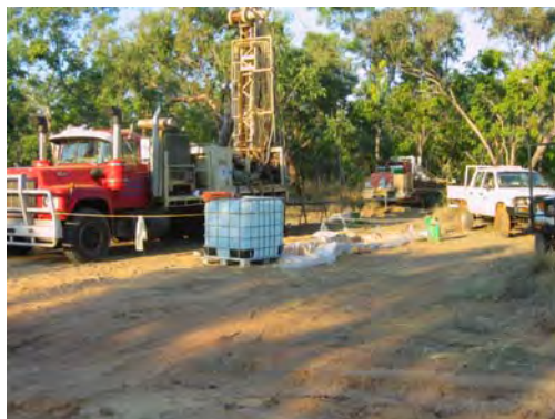
PHOTOGRAPH G4.3 Investigator Mark V drill rig on MACK truck at Fishers Ridge. Trailer with drilling supplies (drill rods, sand gravel, standpipe etc) behind rig
