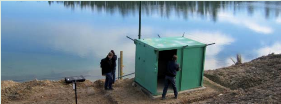
Remote monitoring station at the Benambra tailings dam. Source: Victorian Department of Primary Industries.
