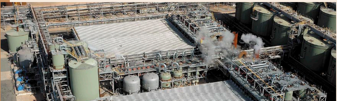
Digestion units at Comalco Alumina Refinery (shown as tubes) where a focus on water efficient design means that the tubes contain process water and heat rather than losing both through dissipation from open tanks.
