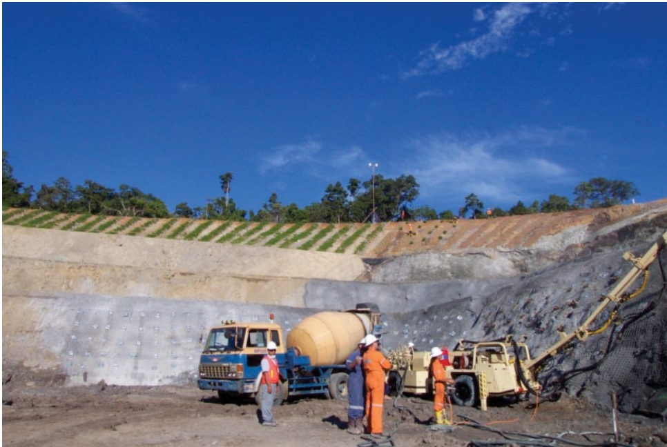
Figure 1.1 - Progressive rehabilitation of the box cut (background) during portal construction at Newcrest's Kencana mine, Indonesia.
