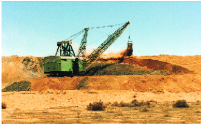
Photo: Optima Energy Using old page dragline to adjust slope and cover with topsoil (note smoke on left side of photograph).
