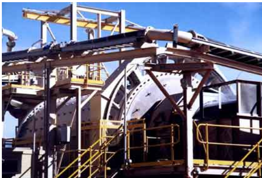
The optimised crushing circuit. Photo Courtesy of Newmont Australia
