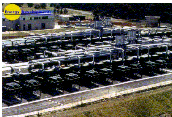
Waste methane power generation unit at Appin Photo courtesy of BHP Billiton Appin
