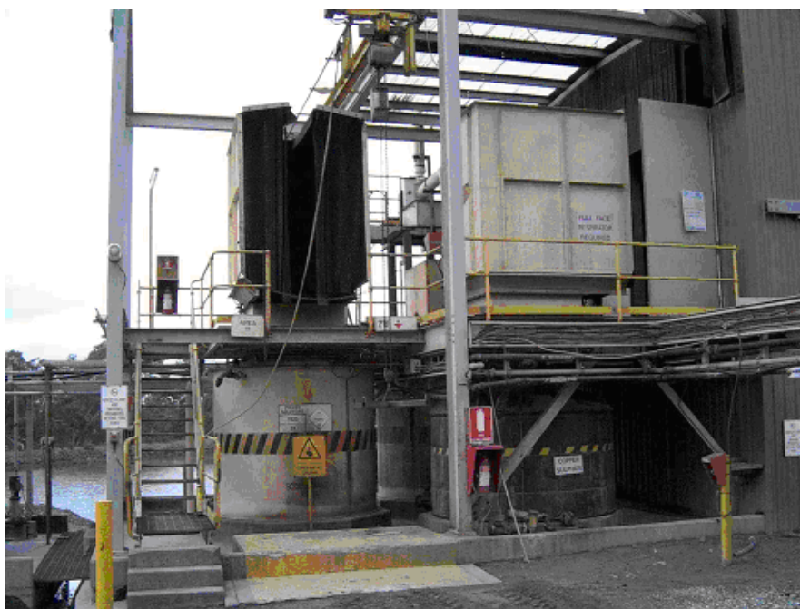
Cyanide mixing area. Level meter, safety equipment, and emergency button are all clearly labelled and easy to access. Bunding ensures any spillage reports to the secure process water pond (photo Stawell Gold Mine Pty Ltd).
