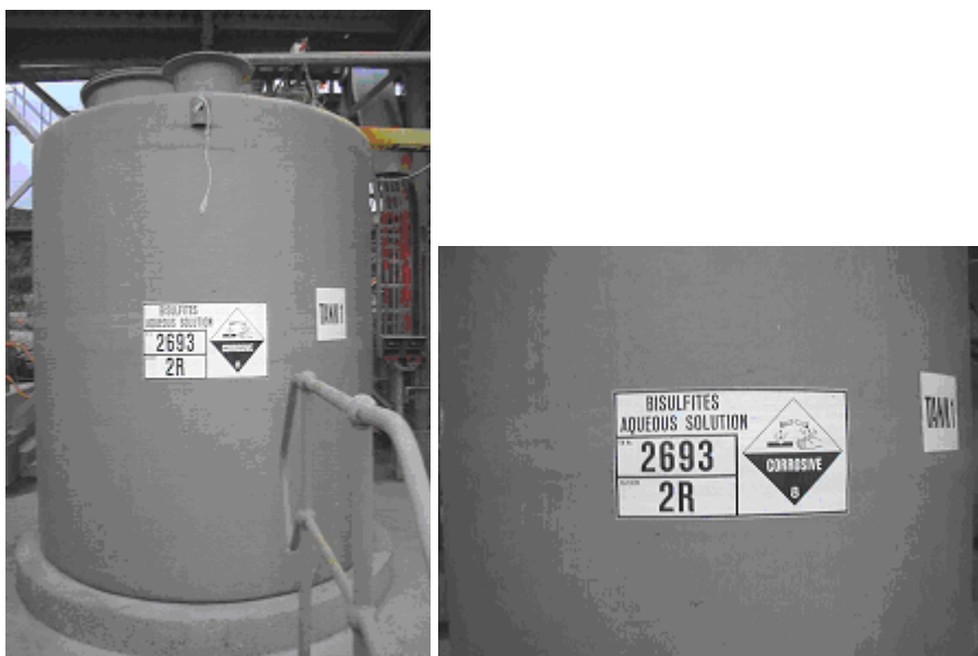
All gold processing reagents (such as sodium bisulfite) are stored in an undercover bunded area. Cyanide packaging is returned to the supplier as part of the supply contract (photos: Placer Dome Asia Pacific - Henty Gold Ltd).
