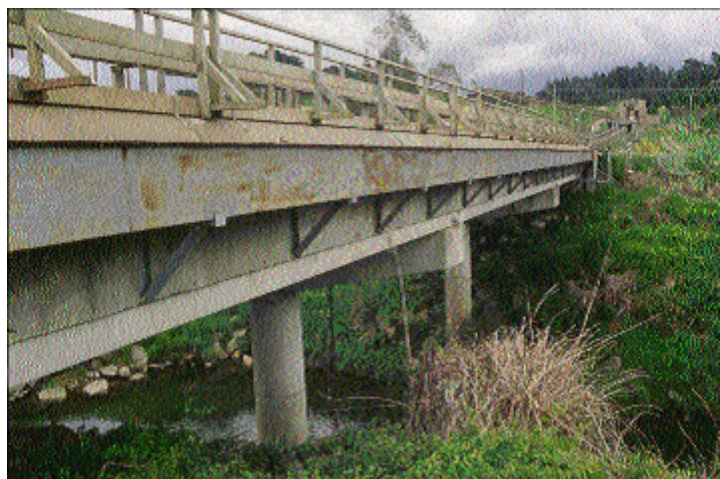
Tailings line crossing the Ohinemuri River (Photo: Waihi Gold Mining Company Limited)
