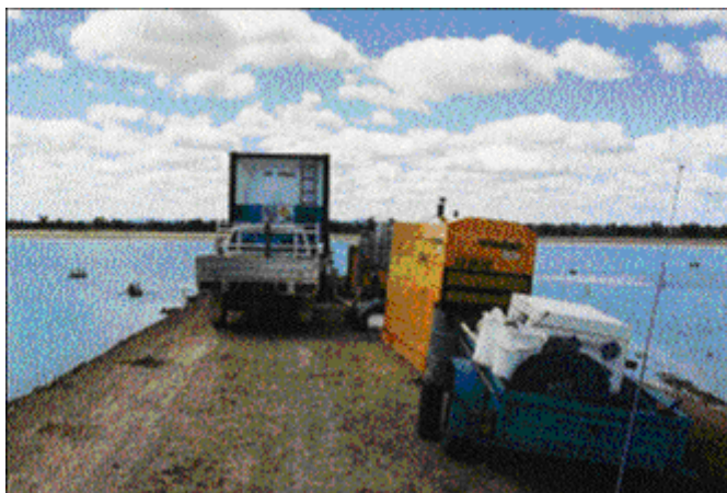
Tailings Dam No.1, Hydrogen peroxide dosing equipment on the central causeway. Photo: North Limited
