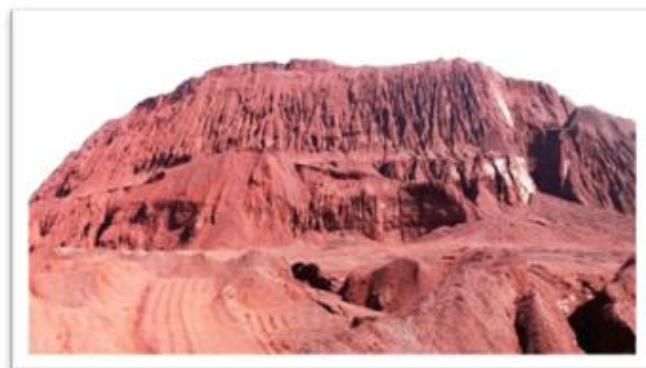
Fig. 2: Slope failure in Fines dump
