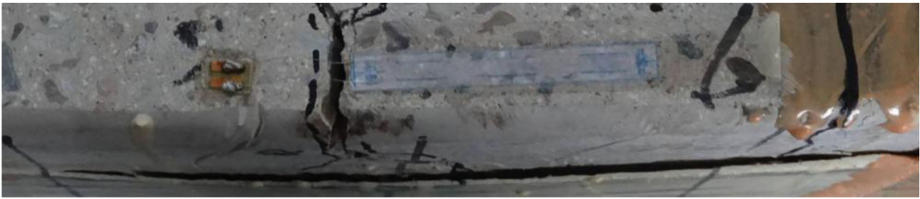
Fig. (20). JM-2 CFRP debonding breakage.
