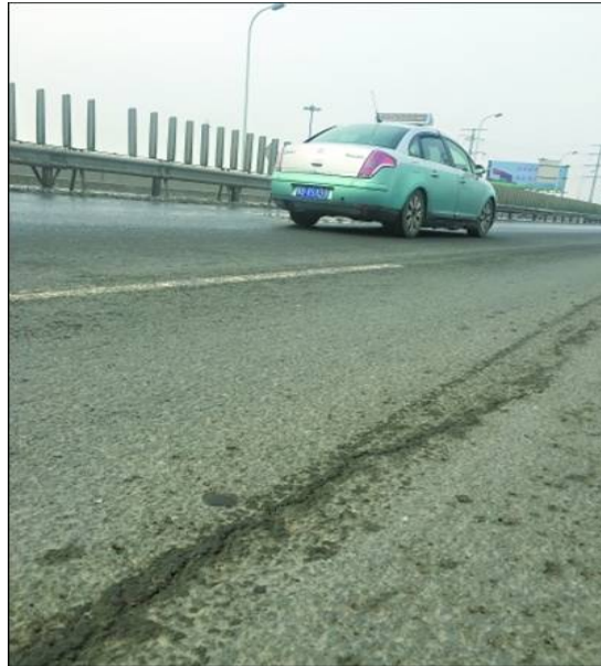
Fig. (1). Vertical cracks on the Baishizhou Yangtze River Approach-Bridge
