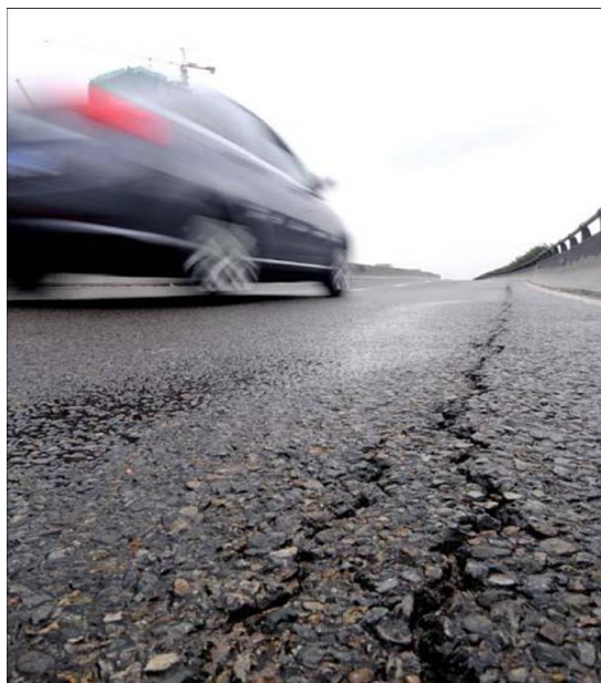
Fig. (2). Vertical cracks on the liming high level bridge in Fujian province.
