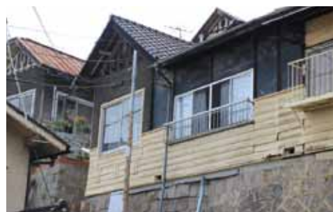
Onomichi City: Renovation project for empty houses (renovated house "Saka-no-ie") through cooperation between the public and private sectors
