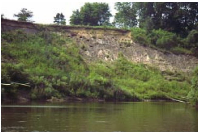
Figure 4.3 Eroding Bluff near Delaware
