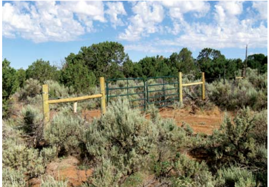
One aspect of the Conservancy's management plan was repairing the perimeter fence and installing a gate.
