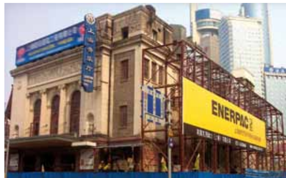
Two high-profile Chinese projects involved moving the Shanghai Concert Hall and (center) positioning the roof on the Bird's Nest Olympic Stadium.
