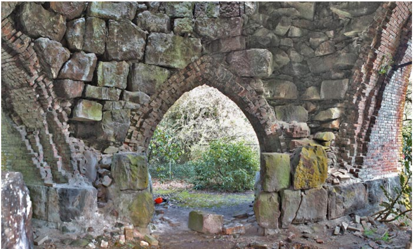
Panoramic view of the interior shows where large blocks have fallen and exposed the rubble fill between the inner and outer walls. Photo/Frank and Susanna Kuo
