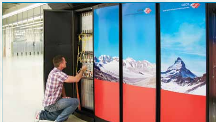
Tödi, the Swiss National Supercomputing Centre’s 137-teraflop XK6 Cray supercomputer, is the first GPU/CPU hybrid supercomputing system. Image credit: Michele De Lorenzi/CSCS
