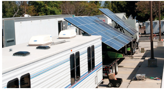
“The Mentalist’s” solar panels in action powering base camp while on location in the City of Industry, California.
