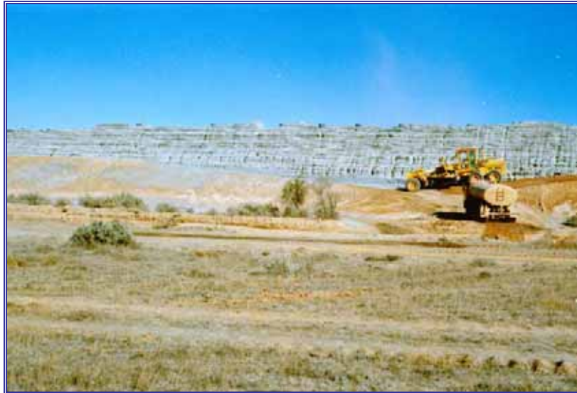
Fig. 34. Excavating material from borrow pits, with the tailings impoundment directly behind, 1981. (Source PIRSA 049699)
