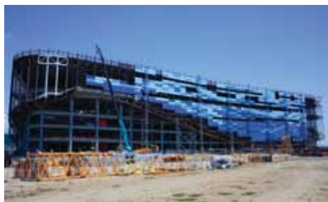
Construction on Sochi's figure-skating and short-track center is shown in this photo dated June 7. (Sochi 2014) ▲
