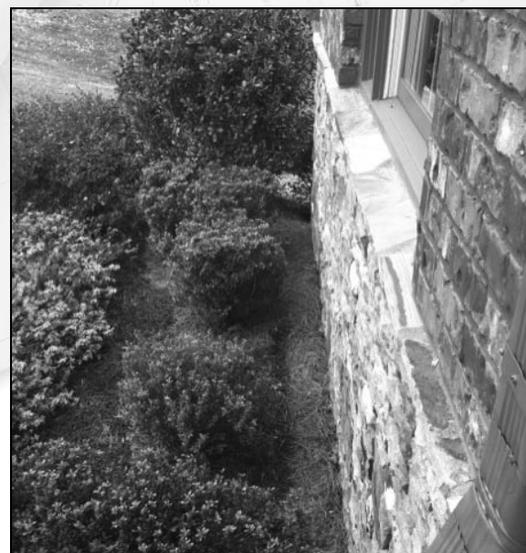
Shrubs around your home are part of the quality landscaping of your lawn, but care must be taken to keep them a good distance from foundations.
