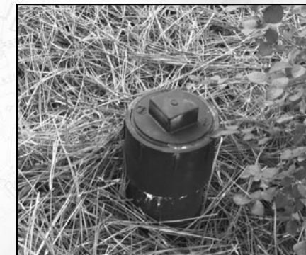
If you have a septic system, a 4" PVC sewage clean out may be located outside your home.
