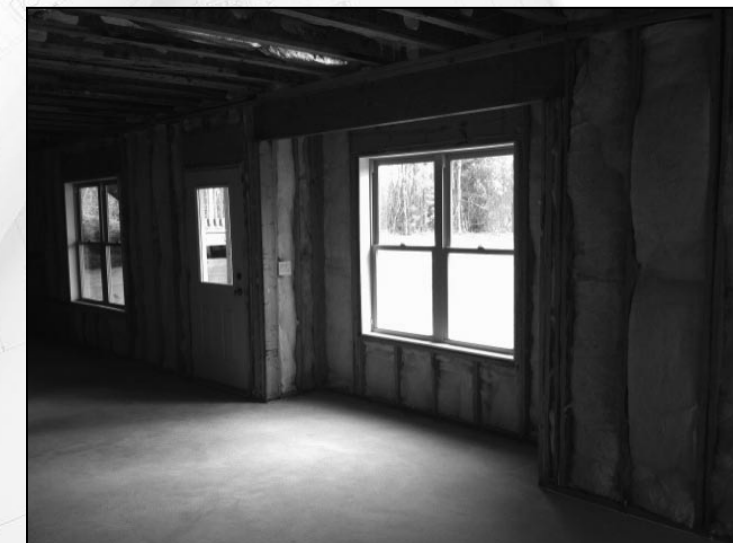
Fiberglass insulation protects most of your home from hot and cold elements. Blown insulation, wall sheathing and duct work or piping insulation protect other areas.
