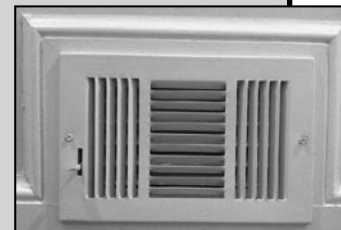
Registers in each room allow you to adjust the air flow in different areas of your home.
