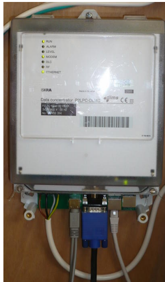
Figure 20: Iskraemeco P2PLC data concentrator at Delta
