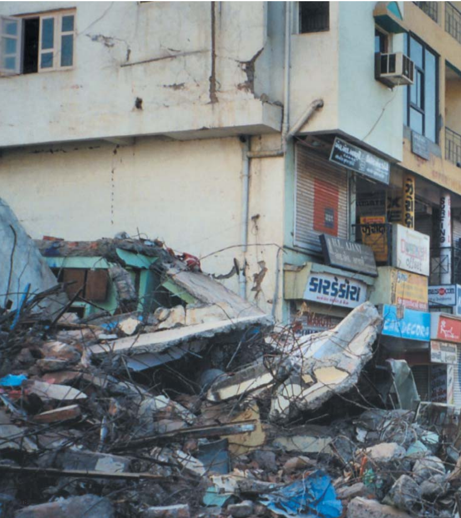
20 A row of houses in Bhuj after the earthquake on 26th January 2001.
