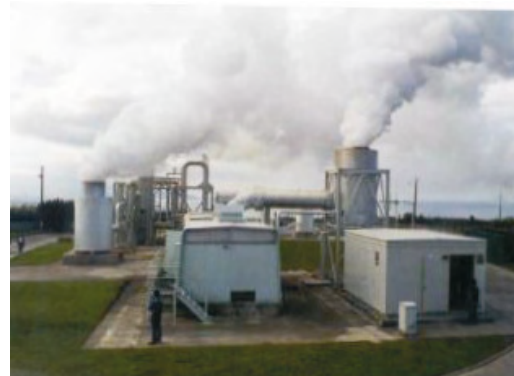
Fig. 8.48 Direct-intake, non-condensing single flash geothermal power plant at Pico Vermelho (São Miguel Island, Azores) exhausting steam to the atmosphere. (source: [2004Lun b ]).
