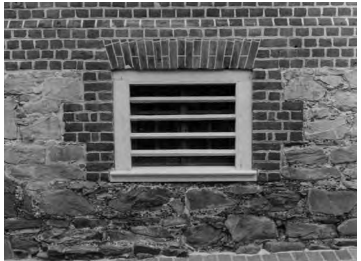
Figure 79. Detail of William Paca House foundation and cellar window. The all-header brick bond and the pebbles in the stonework mortar joints (galleting) are distinctive Annapolis details which require skilled craftsmanship to preserve.
