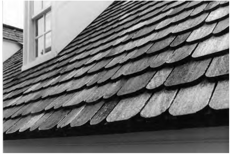
Figure 81. Detail of sawn shingle roofing, west dependency of the William Paca House.
