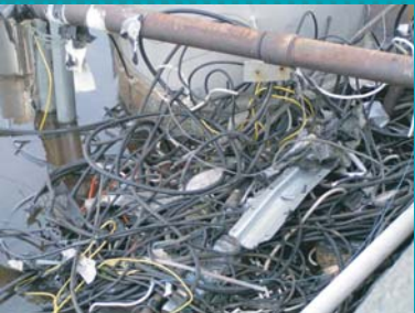
Damage caused by rooftop transmitter installation
