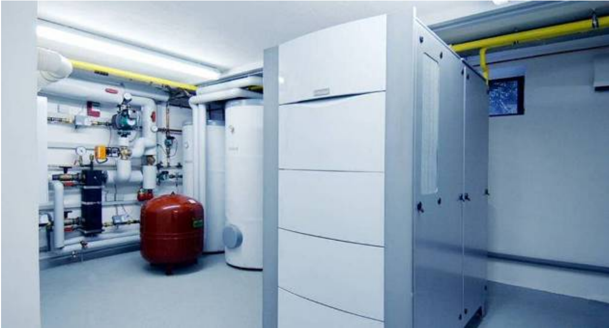
Figure 9: Field test system in Baunatal near Kassel (Germany)
