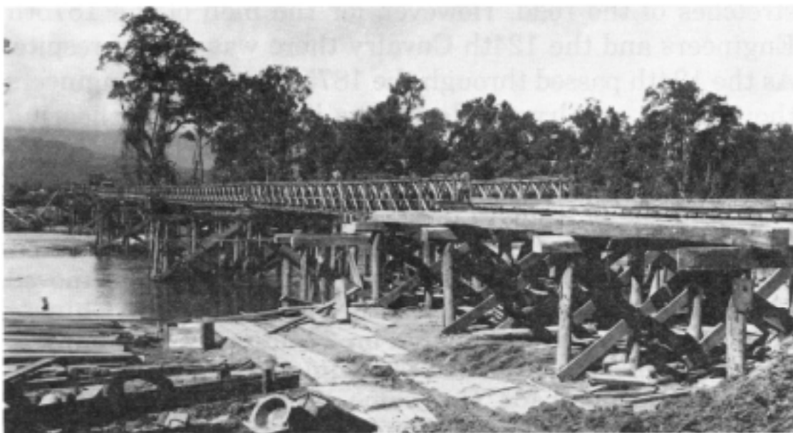
Construction of a Bailey bridge over the Mogaung River south of Warazup, Burma.
