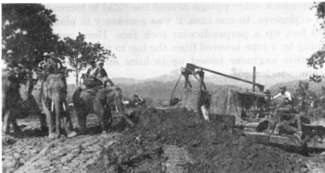
Survey party on elephants passes a bulldozer on the Ledo Road in the jungles of north Burma.
