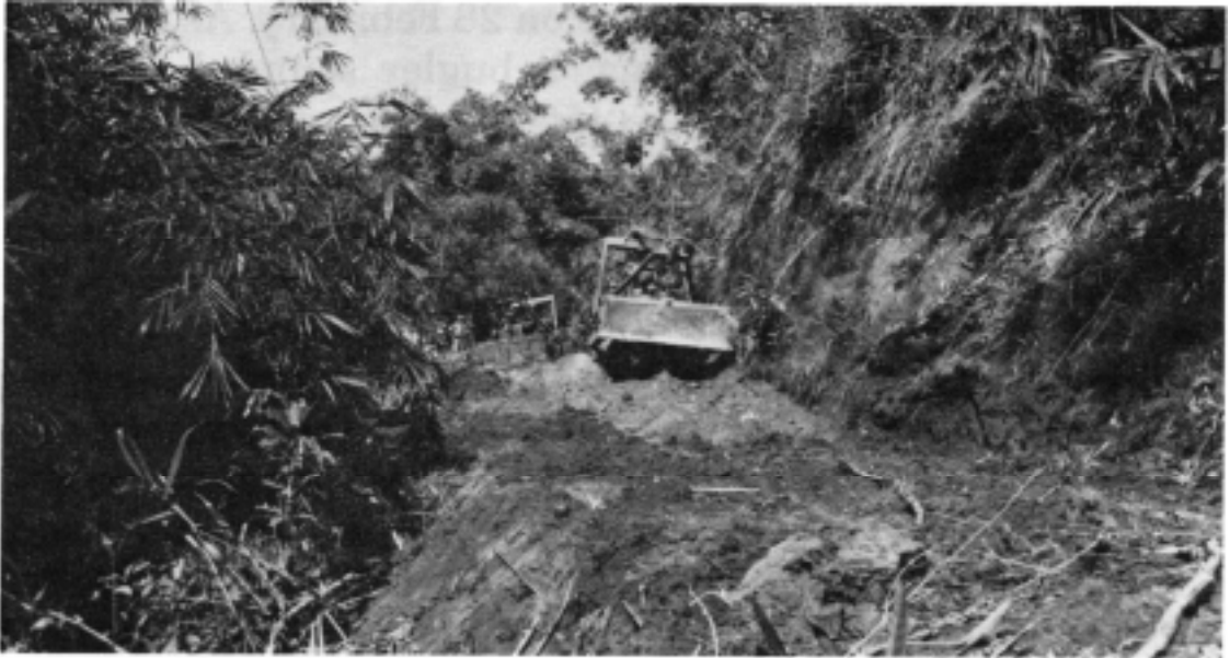
Bulldozers clear a slide in Burma, as engineers construct the Ledo Road.
