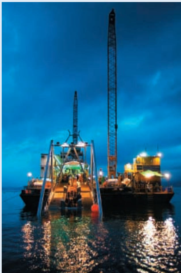
Submarine pipes have been laid in preparation for the delivery of natural gas from Guangdong LNG terminal to Hong Kong and China Gas Production Plant in Tai Po.
