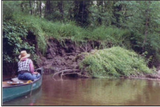
Undercutting of the toe eventually results in huge sections of River bank collapsing into the channel.
