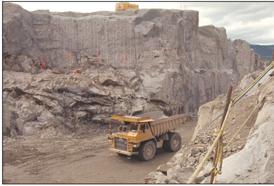
Site of the 77 m-high Toulnostuc concrete-faced rockfill dam in Québec, which went ahead recently.
